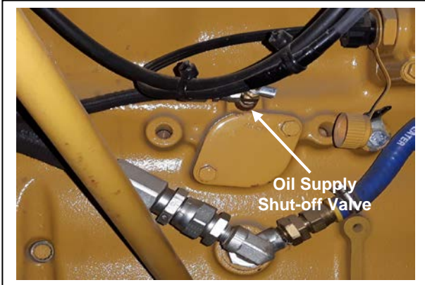
Picture 5 (Oil supply Shut-valve- C32)
