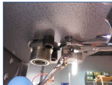
7) Slightly unscrew fitting- as required to orient fitting facing forward (or in direction required for install), then use (2) wrenches to hold fitting in place while tightening locknut
